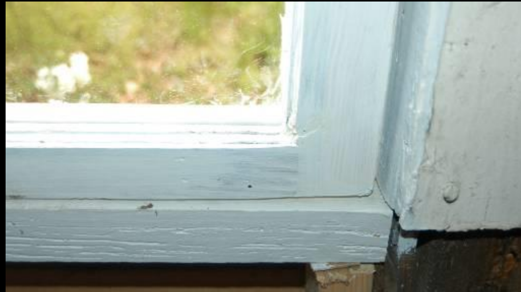
Primed window after deteriorated bottom rail and bottom of stile were repaired.
