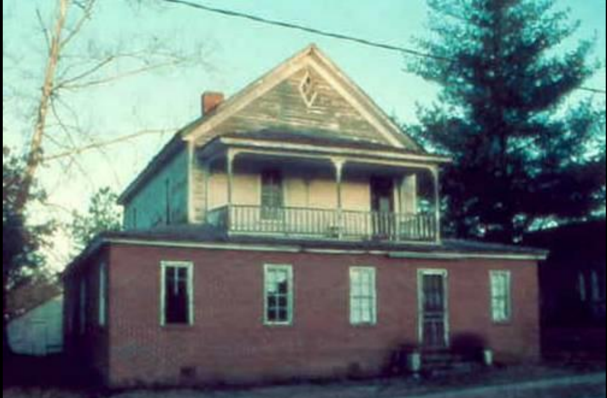
This old addition was off of the front of the building and resulted in the loss of part of the front porch. The addition does not complement the historic house as it is made of brick instead of wood and the orientation is different.
