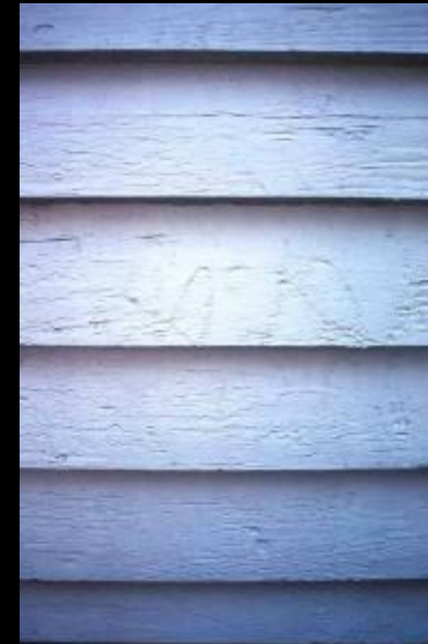
The damage from a pressure washer is still visible after painting
