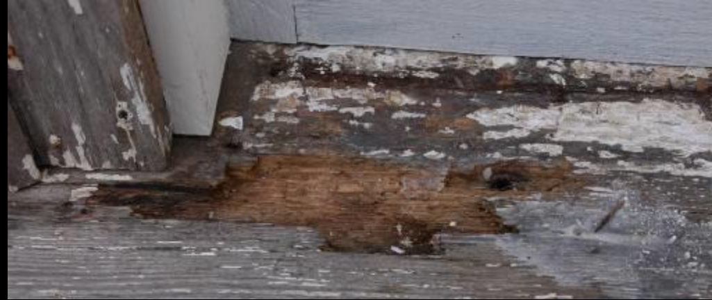
Remove deteriorated material, kill wood feeding pathogens, repair with epoxy, prime, and paint.
