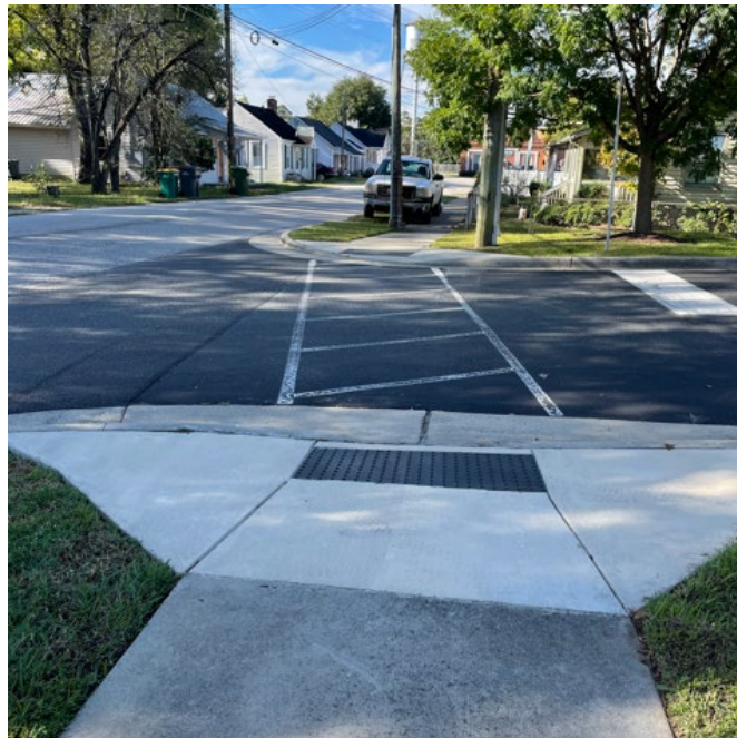
Installation of curb ramps with Detectable Warning Surface at the Municipal Parking lot on Trade and Main St.
