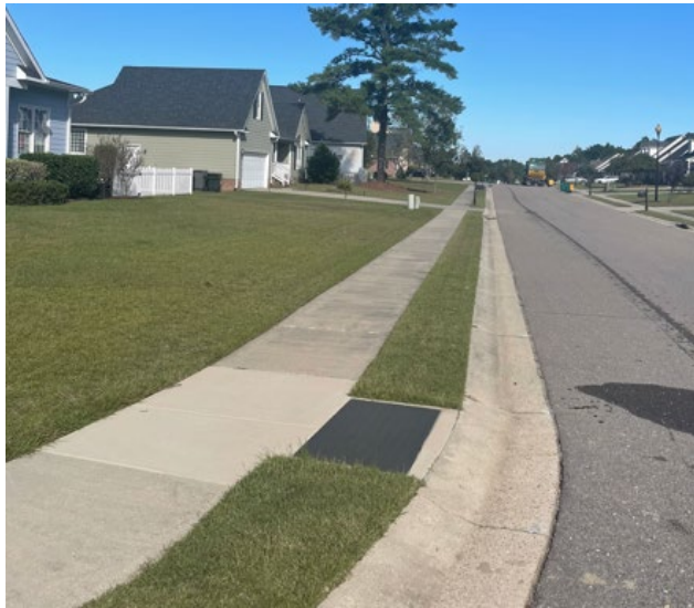
Installation of curb ramps with Detectable Warning Surface through the entirety of Kensington Village
